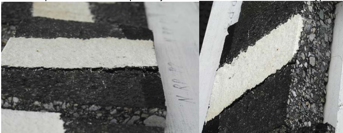
Figure 22: Detailed of thermal stress-cracked asphalt.
