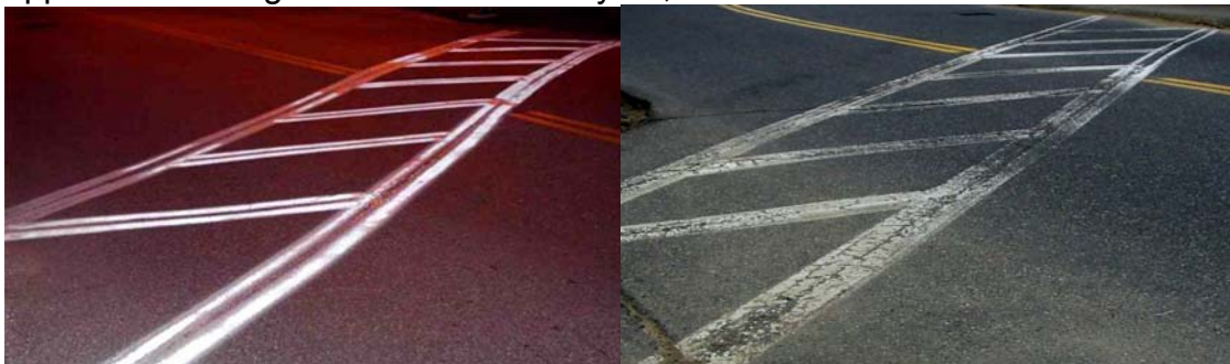
Traffic paint at the Durham test site. Left on August 2002. Right on May 8 th , 2003.
